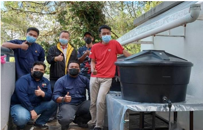
Copthorne Cameron Highlands’ Maintenance Team successfully set up the hotel’s rainwater harvest system.
